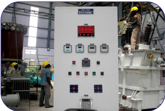
RTCC Panel Assembly
